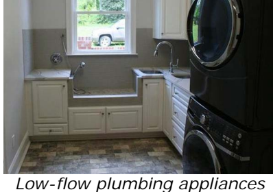
Low-flow plumbing appliances and fixtures, including the pooch's dog wash, reduce water use within the home.
